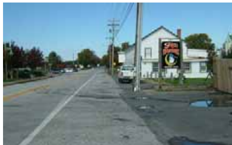
Figure 17 Existing Sidewalk Condition (non-existent)
